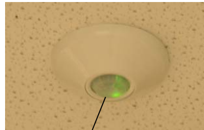
Occupancy Sensor in bathroom
